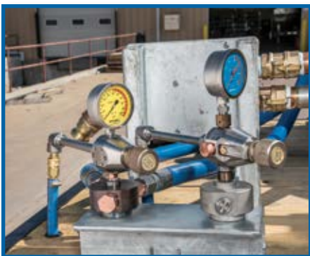
Dual Pressure Control Station
